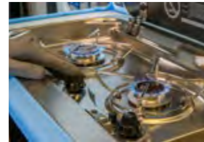
Test on operation of the gas pipes.
